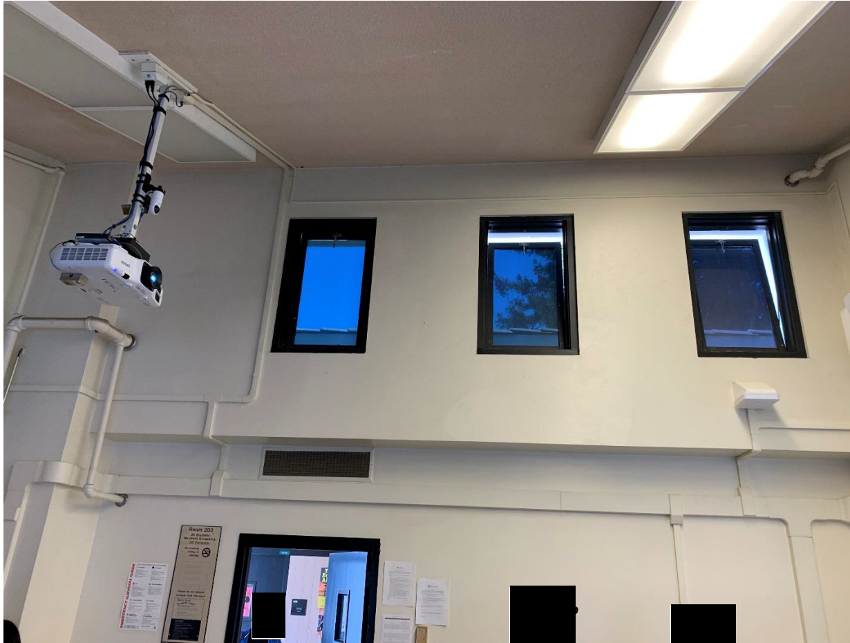
Unsecured Projector, Clerestory Windows in Second Floor Classroom
