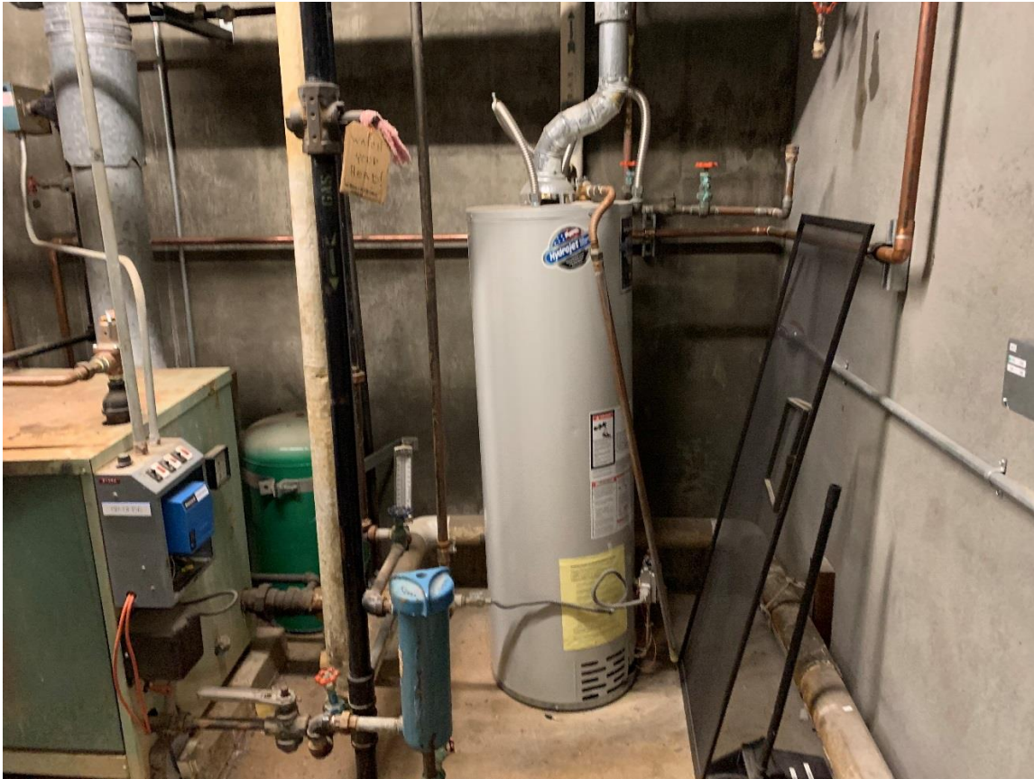
Mechanical Room in Basement of 1985 Addition, Unanchored Water Heater (right), Anchored Green Tank (left)
