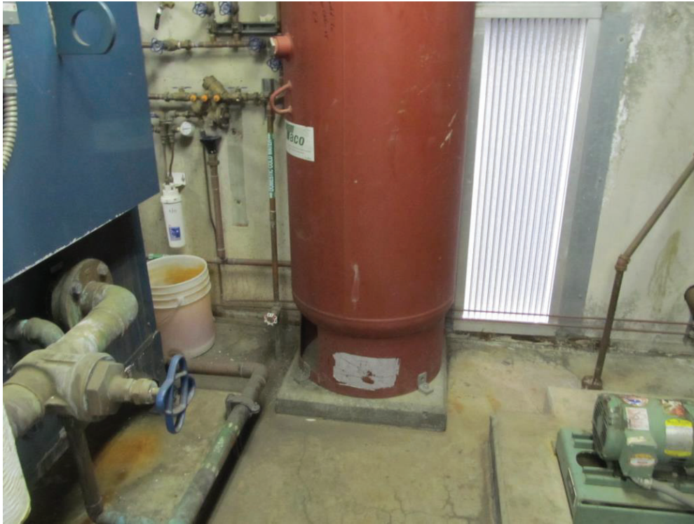
Anchored Tank at Mechanical Room
