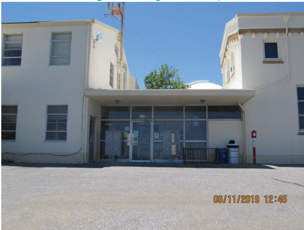
North Elevation of Canopy (Two-story Portion at Left, Canopy at Center, CAAN 7240 Provides Support at Right, Looking South)
