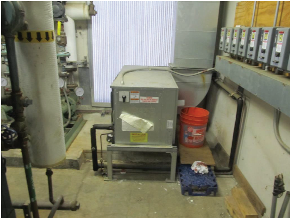
Anchored Equipment at Mechanical Room
