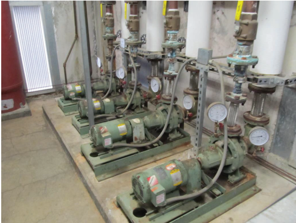
Anchored Pumps at Mechanical Room
