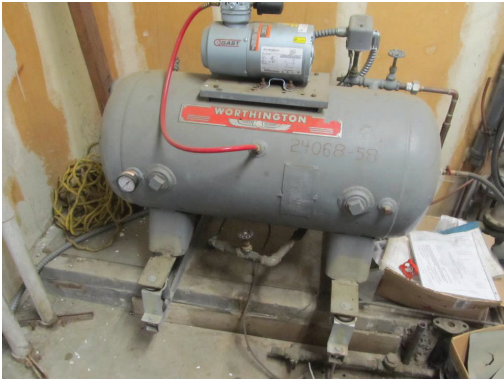
Poorly Anchored Tank at Mechanical Room
