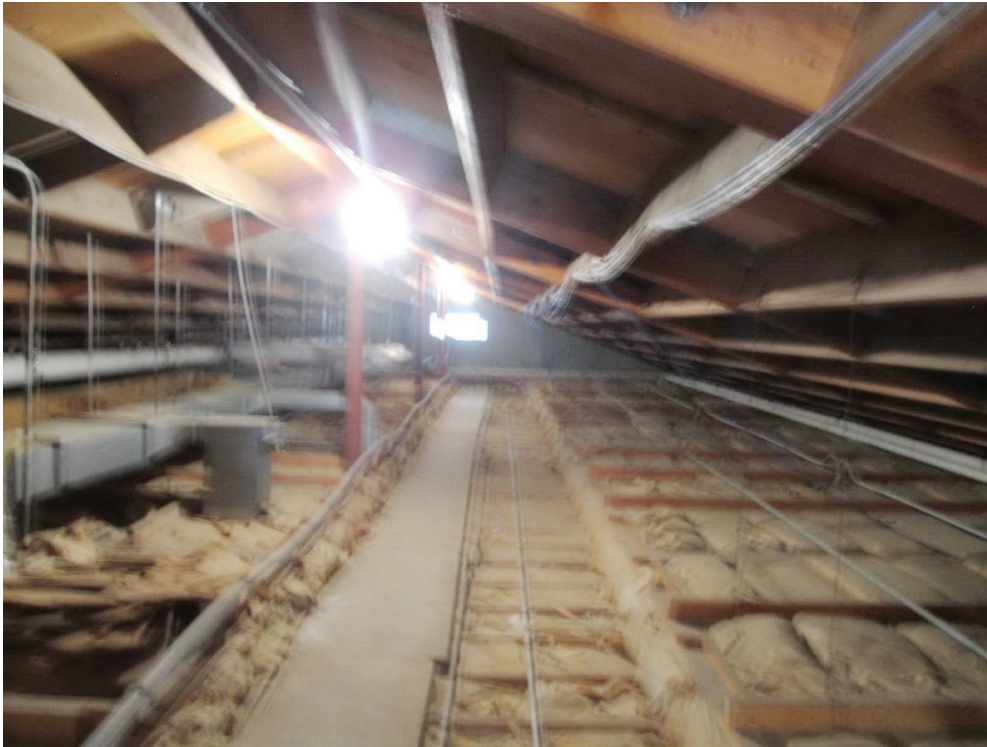
Attic Space Showing Wood Framing at Top and Ceiling Framing at Bottom (Looking West)
