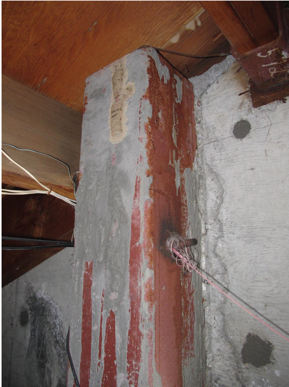
Steel Column Filled with Concrete Attached to Tilt-up Panel in the Attic
