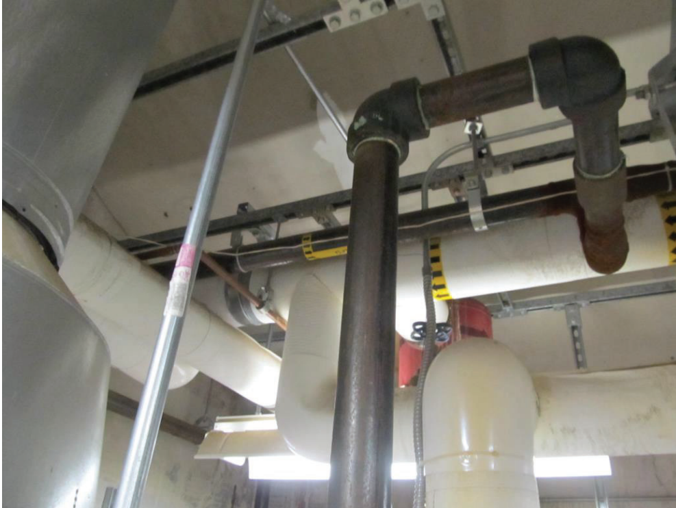
Braced Piping at Mechanical Room
