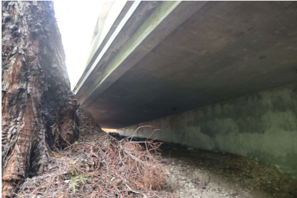
North side of building, looking east. Foundation wall below Level 1 and cantilever slab at Level 1
