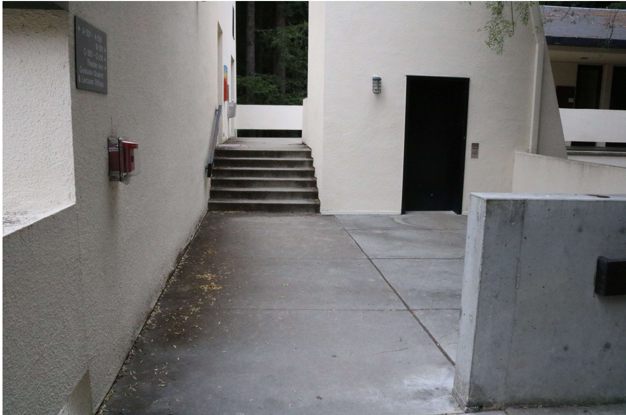
Walkway at east side of building (building to the left, elevator structure to the right)
