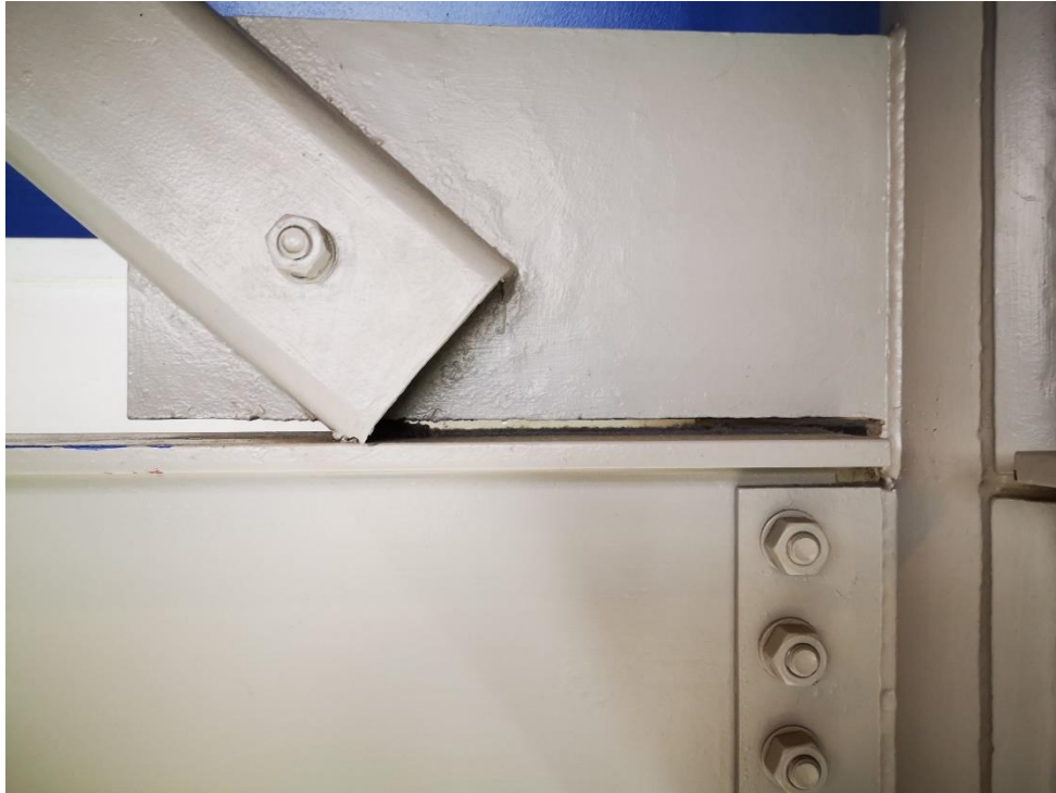
Brace Connection Without Weld at Bottom of Gusset Plate as Shown in Structural Details
