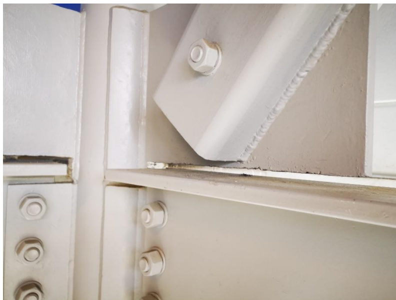
Gusset Plate is Not Welded to the Floor Beam (Second Floor Connection Along Line A, between Lines 1 and 2)
