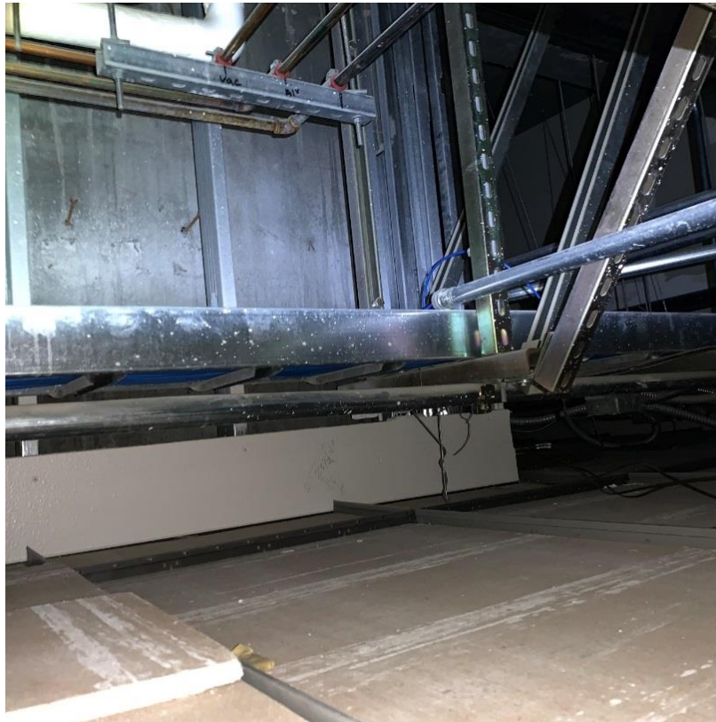
View Above Ceiling at Cable Trays Braced with Unistrut (Corridor Near Building D300)
