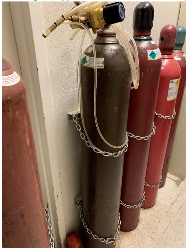
Building C Room C514 (3 Cylinders Anchored to Wall, One Anchored to Dolly, One Unanchored)
