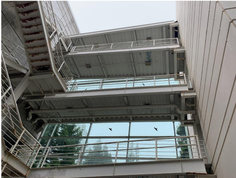
North Elevation of Bridge Upper Portion (Looking South from Courtyard, Building D at Left, Building A1 at Right)
