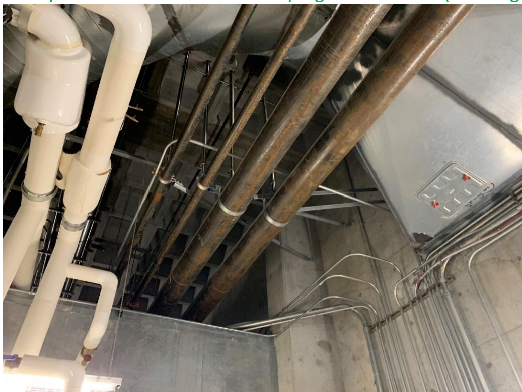
Laterally Unrestrained Ducts and Piping at Basement (Building D)
