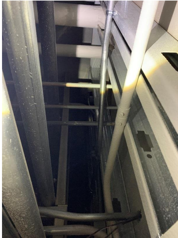
View Above Ceiling in Corridor near D300 with Partitions Anchored at Top (Building D)
