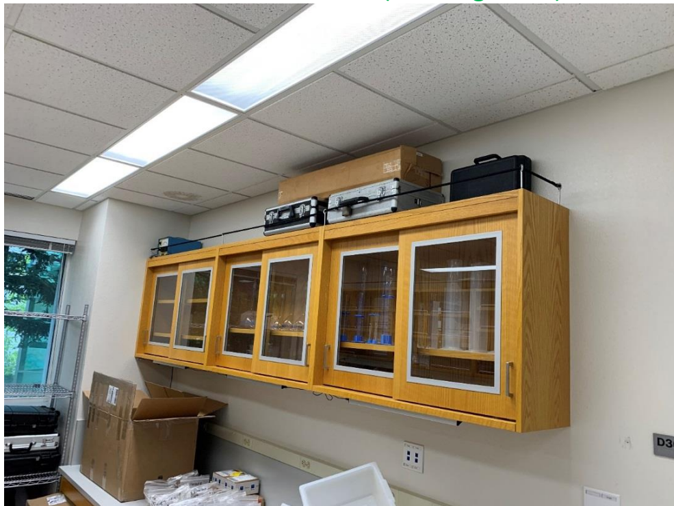
Restraints at Top of Cabinet (Building D360)
