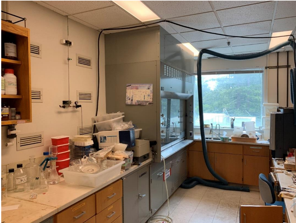
Anchored Fume Hood (Building D360)
