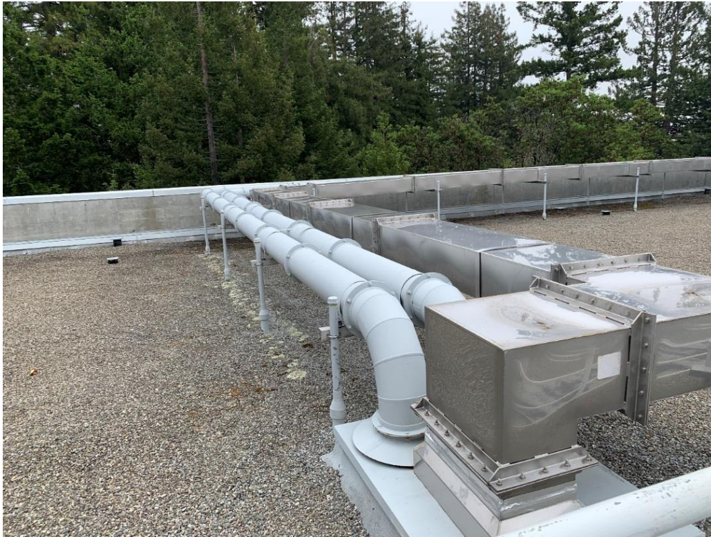
Laterally Unrestrained Pipes at Roof (Building D)
