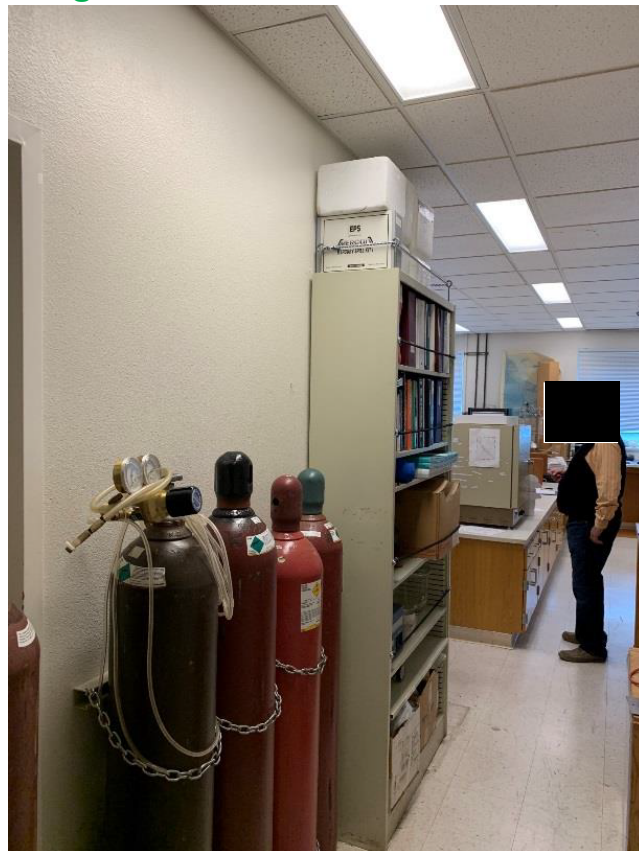
Building C Room C514 Tall Cabinet Unanchored
