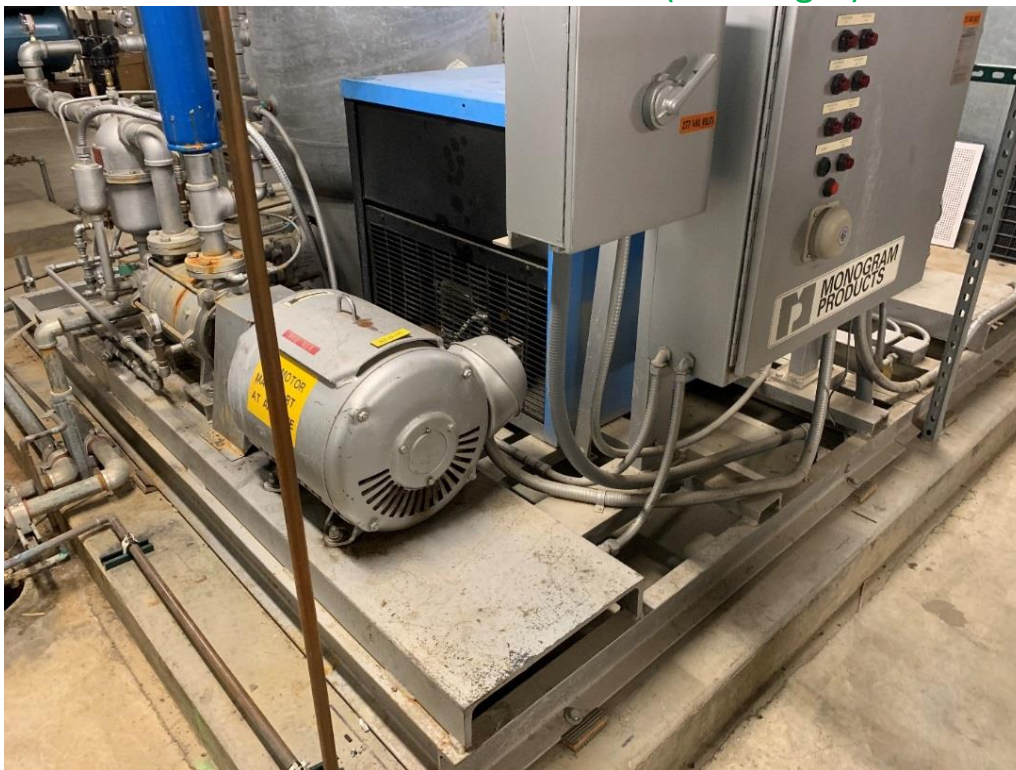
Anchored Equipment at Basement (Building D)
