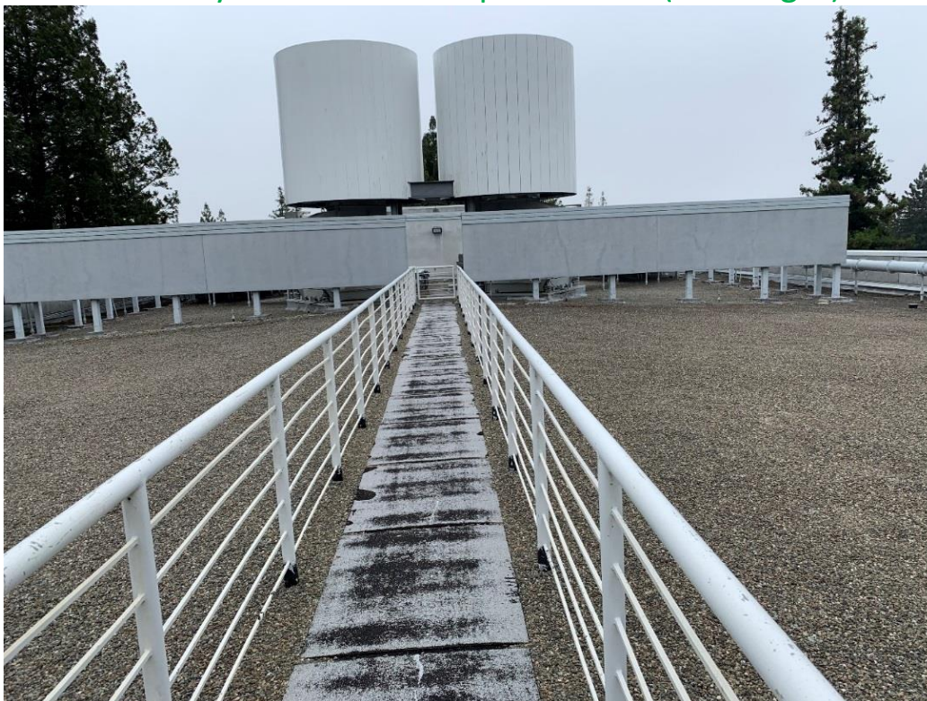
Restrained Cooling Towers at Roof (Building D)
