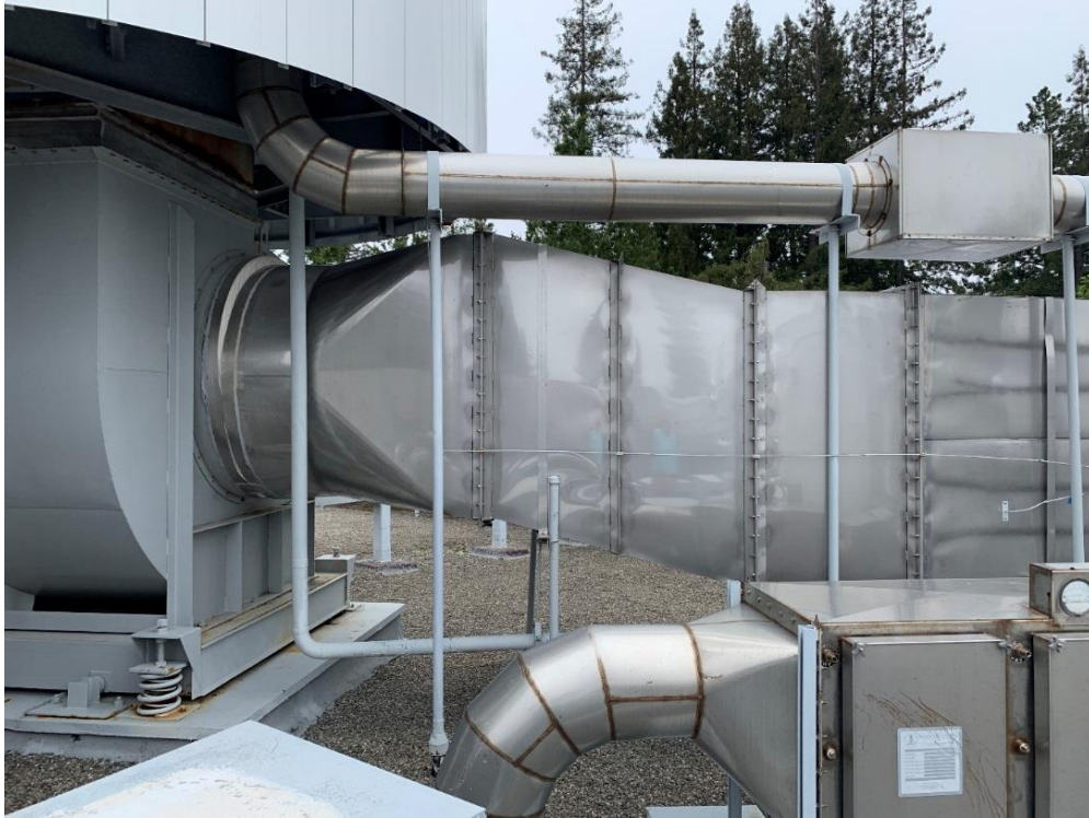
Laterally Unrestrained Pipes and Ducts at Roof (Building D)
