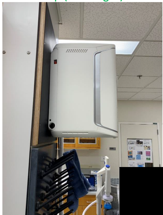
Wall Anchored Milli-Q Tank (Building D360)
