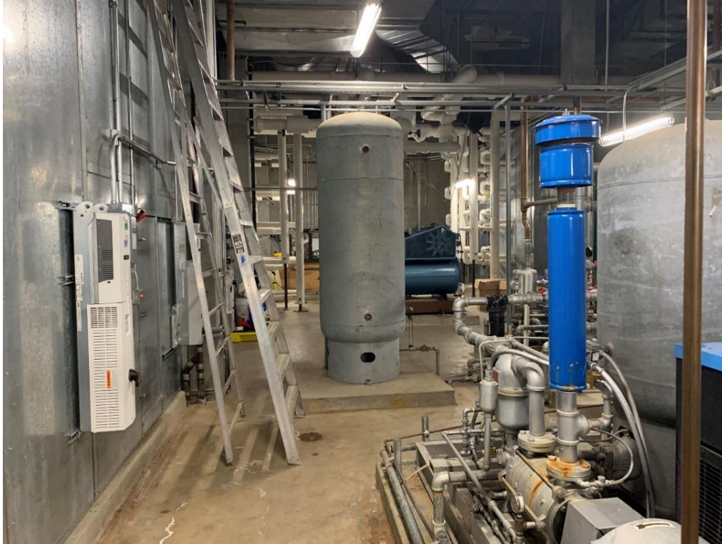
Anchored Tank at Basement (Building D)
