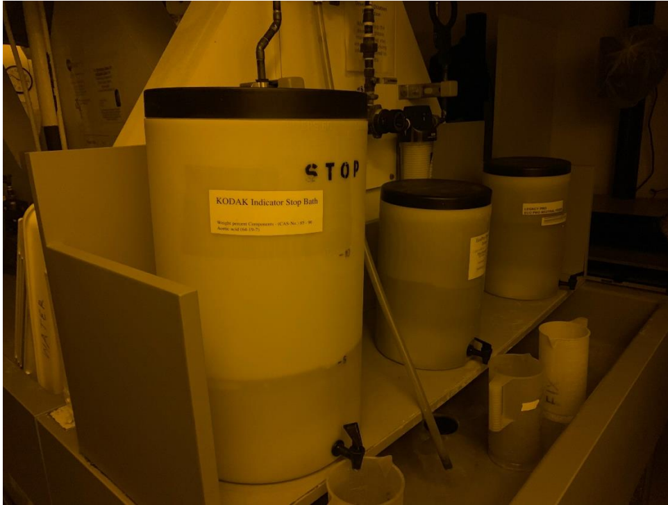
Unbraced chemical tanks in dark room
