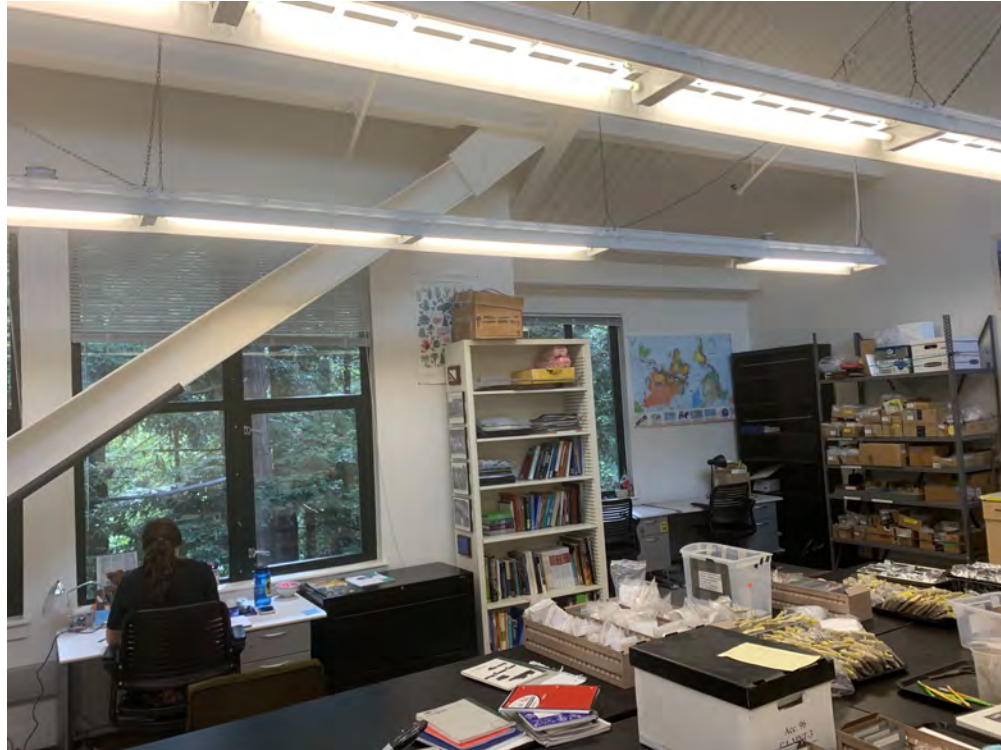
4th floor - Brace not framing into column
