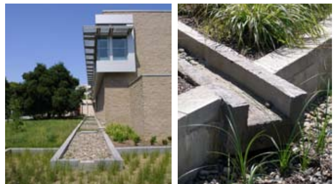
Concrete Stormwater runnels
