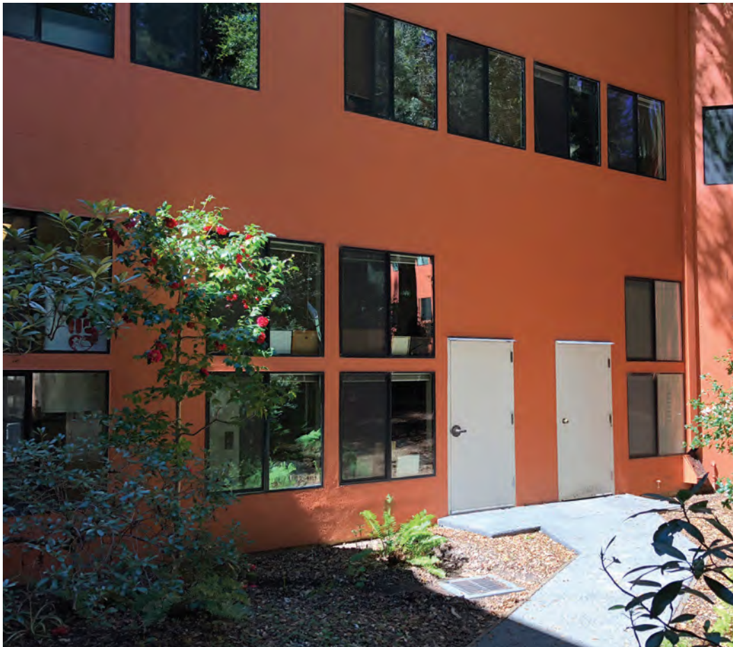
Fig. 2.2-4 Color at windows at landscape-facing facade. Note: Doors should be painted to match facade color
