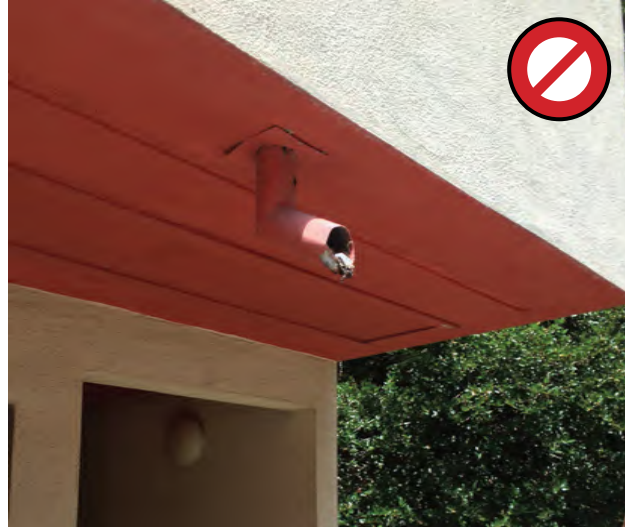
Fig. 3.2.5-3 Existing downspout locations that shall not be utilized in new construction (Left to Right: R4 & R2)
