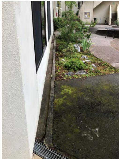
Fig. 2.2-25 Runnel at piazzetta facade (left) and gutters, louvers, and downspouts painted to match building facade (right)
